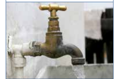
Taps installed in various campus locations
